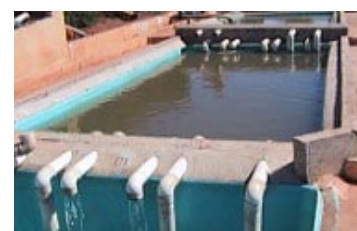
Washing water purification system
